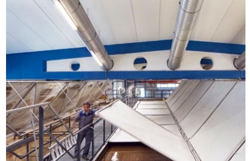
Swarovski water treatment facility in Wattens, Austria
