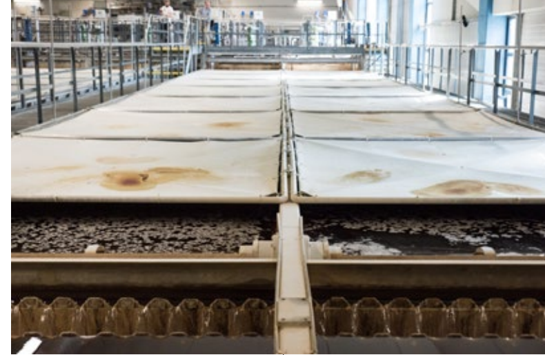
Waste water treatment facility, Wattens, Austria
